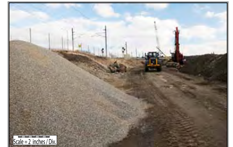
Coarse gravel shown here (#8 - washed 1/2 inch) fills the French Drain, defined above. This view is looking east toward the Niantic River.
